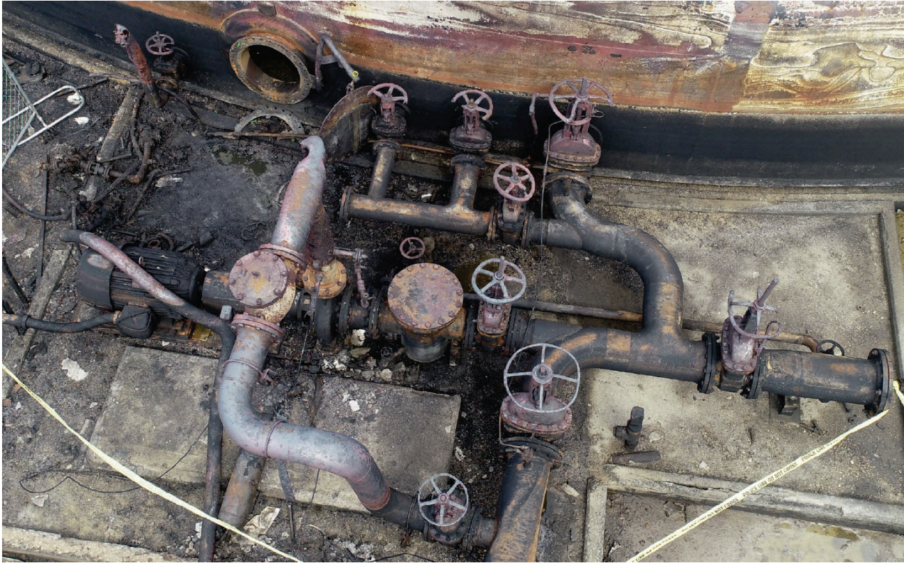
Figure 5. Tank 80-8 Piping Manifold. This photo shows the post-incident condition of the Tank 80-8 piping manifold. (Source: ITC).
