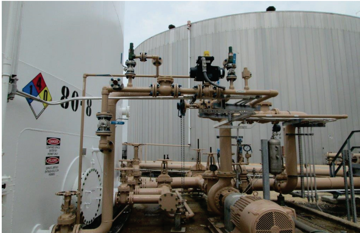
Figure 3. Tank 80-8 Piping Manifold. This image taken before 2016 shows Tank 80-8 and its piping manifold. (Source: ITC).
