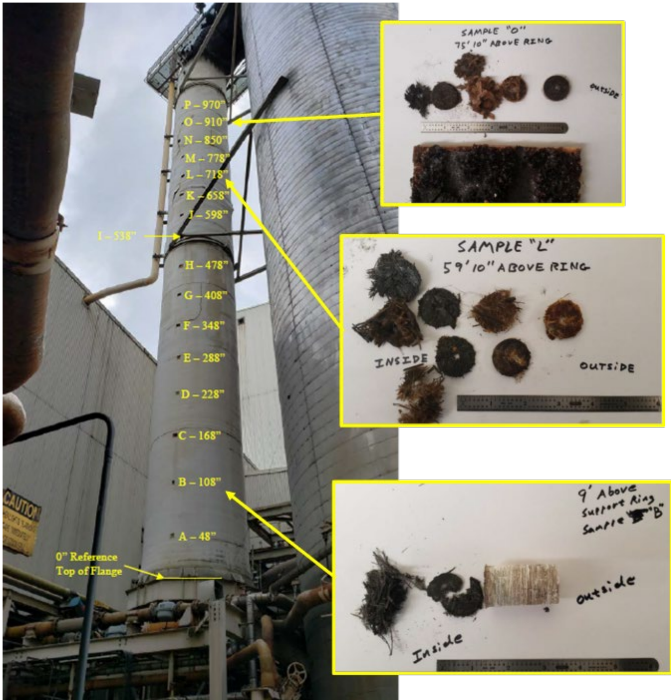
Figure 10. Internal fire damage in the upflow tower. (Credit: Evergreen. Edited by CSB.)
